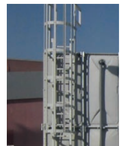
GRP external ladder
