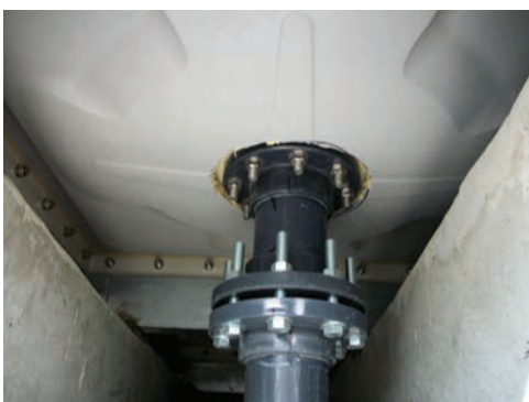
UPVC drain pipe
