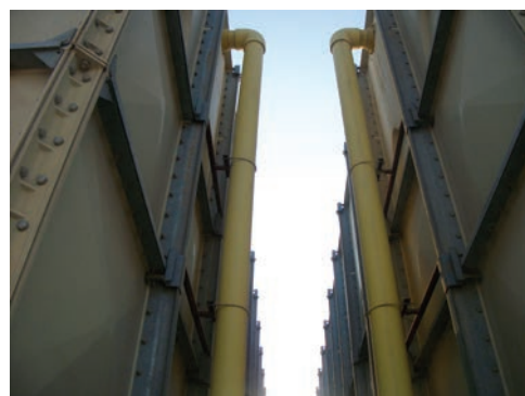
UPVC overflow pipe
