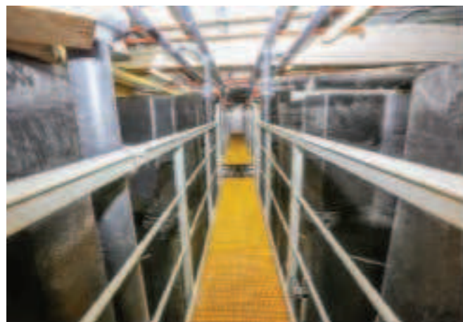
GRP Access to Biofilters tanks
