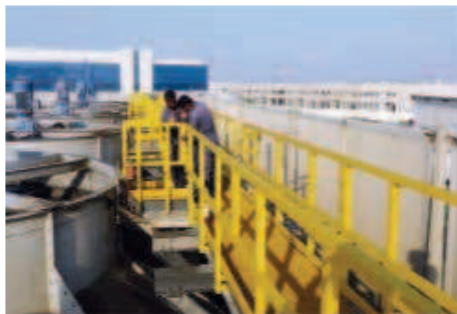
GRP service platform at Emicool DCP at DIP
