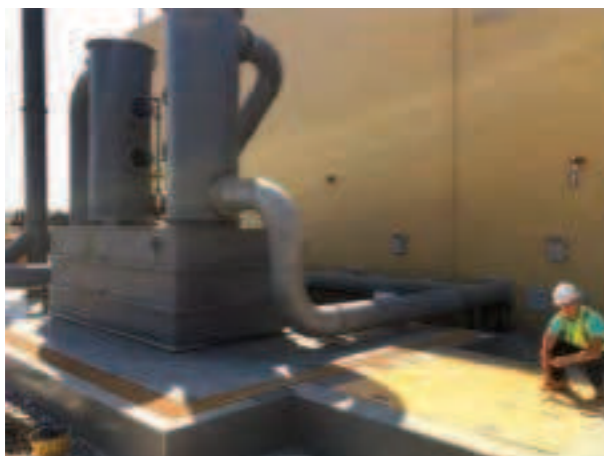
GRP drain grating and cover at Chlorine plant
