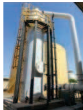
GRP service platform for Odor control scrubber
