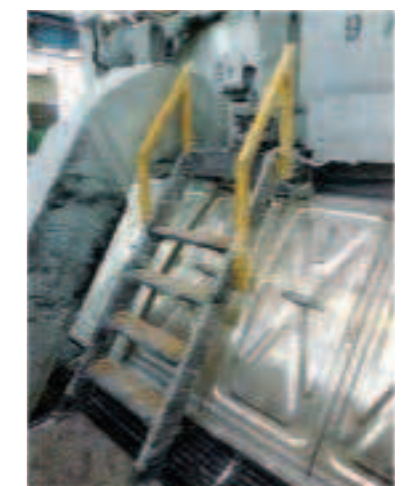
GRP access staircase in Smelter
