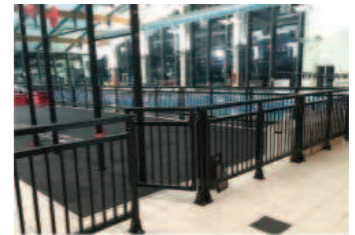
GRP security fence at Swimming pool Hall at Sport city Dubai
