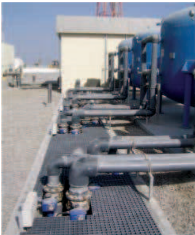
RO Plant at Al Qaffay Island (400m2 Molded Grating)
