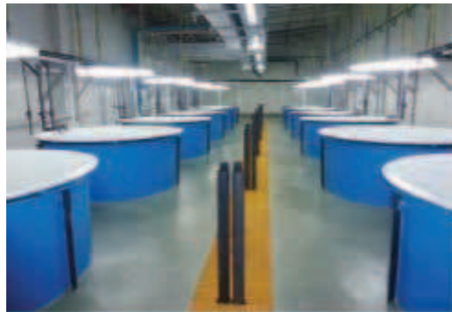
GRP drain grating in Hatchery
