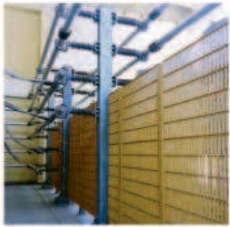
GRP grating fencing 3m High at Qusais Substation
