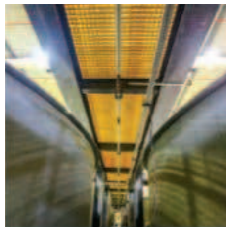
GRP column & beams supports over fish tanks
