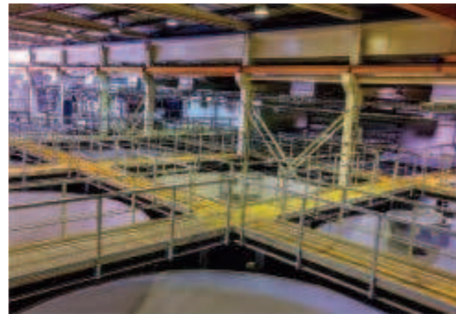
GRP 4 m High grating platforms over fish tanks
