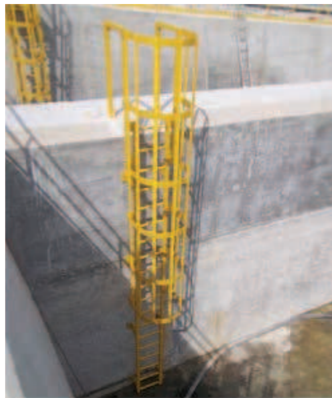
Jebel Ali- Desalination Plant (GRP Safety Ladder outfall area)
