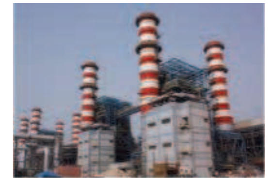
Jebel Ali, 2000 MW power plant Phase M
