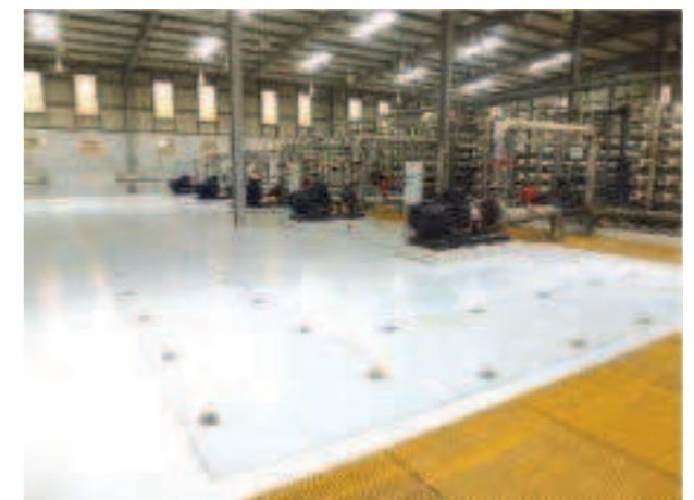
GRP closed chequered cover over Cable trench, Design 5 KN/m2
