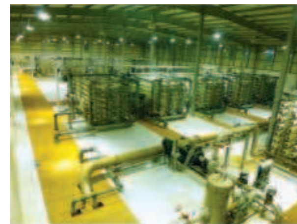
GRP gratings in RO building
