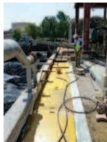
GRP covers at Sludge drying beds
