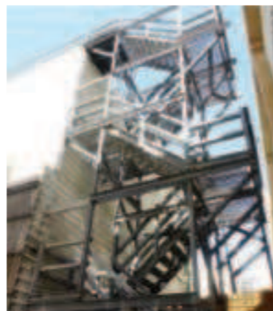
GRP Staircase tower at DCP UAE
