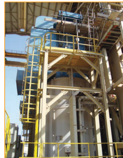
FRP LADDER ON PLATFORM
