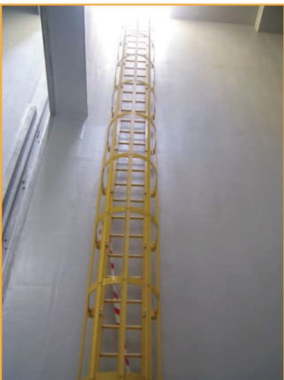
FRP LADDER WITH SAFETY CAGE
